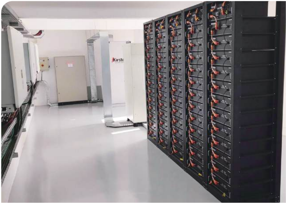
• Brazil 100kW/307kWh PowerRack HV4 Dynamic Capacity Expansion + PV Consumption
