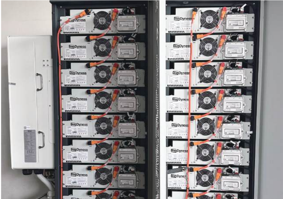
• Bulgaria 112.64 kWh PowerRack HV4F Peak-to-valley Arbitrage+Self-generation and Self-use
