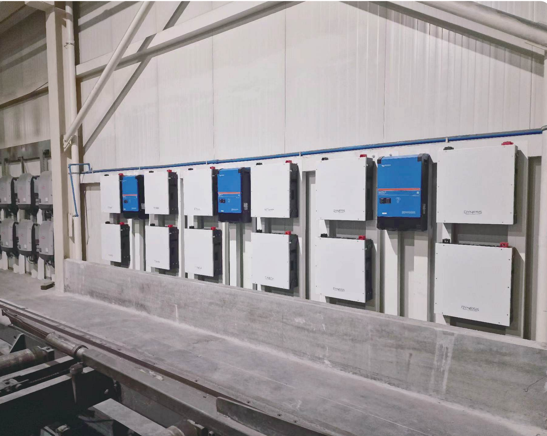
• 61.44kWh 12 units DL5.0C Spain
