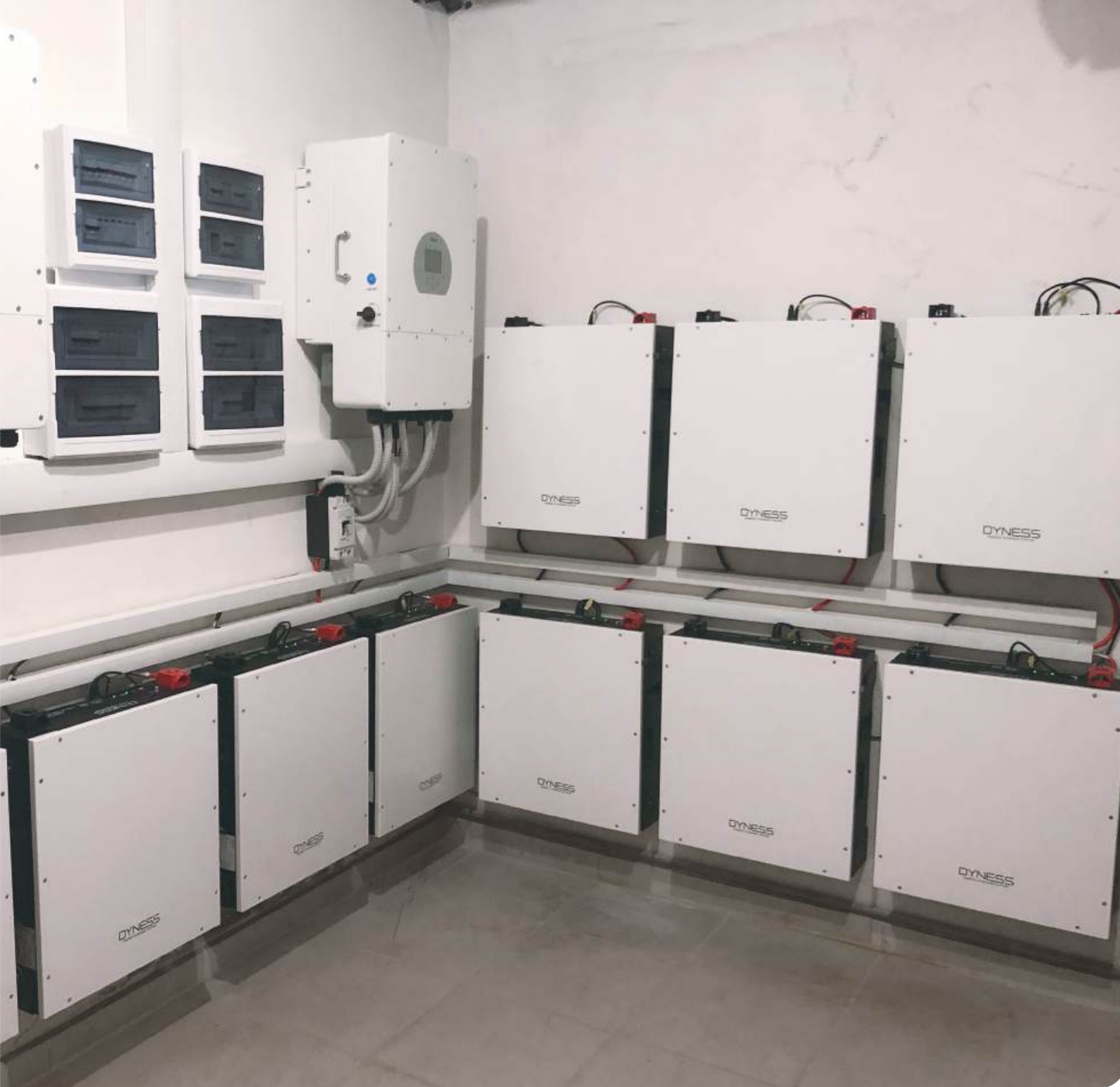
• 48kWh 10 units A48100 Lebanon
