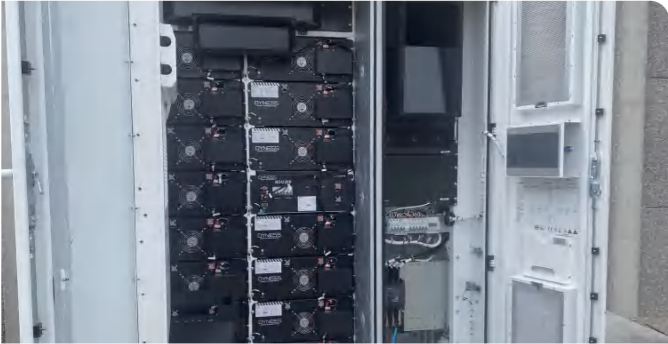
• Belgium DH200F 100kW/215kWh Dynamic scaling (peak-shaving) + PV consumption (self-shaving)
