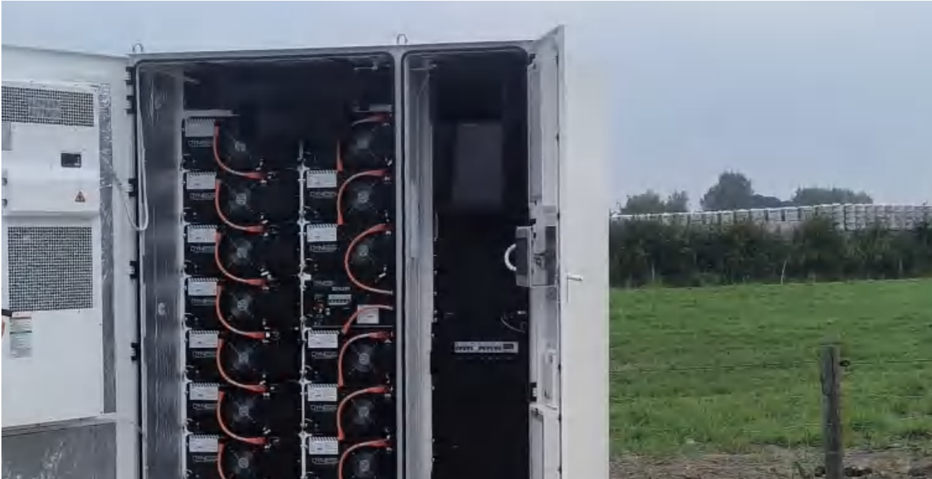
• The Netherlands DH200F 100kW/215kWh Photovoltaic consumption (self-use)
