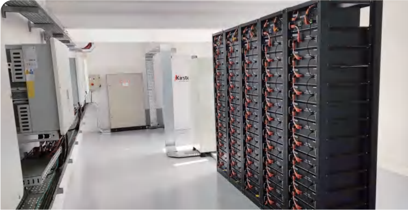
• Brazil PowerRack HV4 100kW/307kWh Dynamic Capacity Expansion (peak-shaving) + PV Consumption
