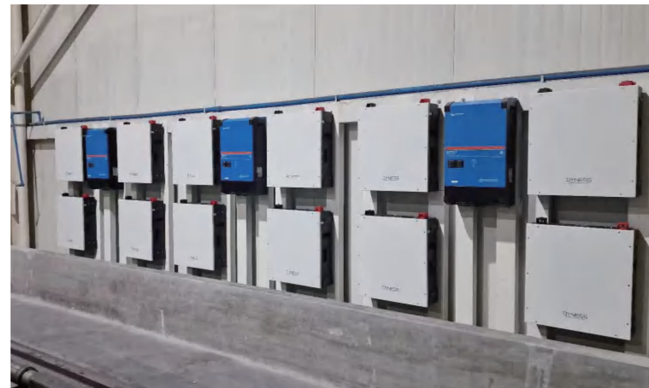
• 61.44kWh 12 units DL5.0C Spain
