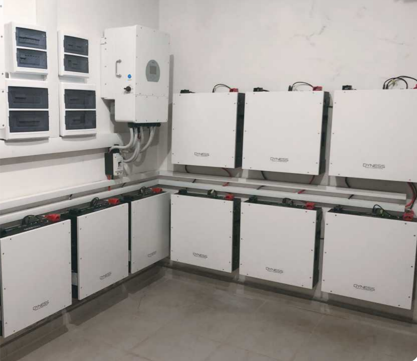
• 48kWh 10 units A48100 Lebanon
