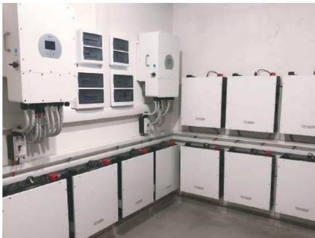
• 48kWh 10 units A48100 Lebanon
