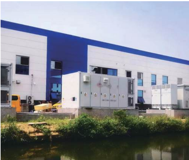
• China 5MW/18MWh DH200F Peak-shaving+PV consumption
