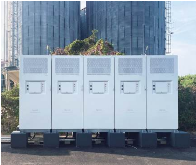
• Spain 500kW/1160kWh DH200Y Self-generation and self-use+PV consumption
