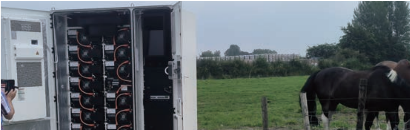
• The Netherlands 100kW/215kWh DH200F PV consumption (self-use)
