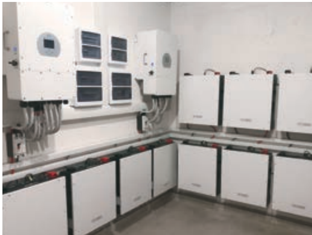
• 48kWh 10 units A48100 Lebanon
