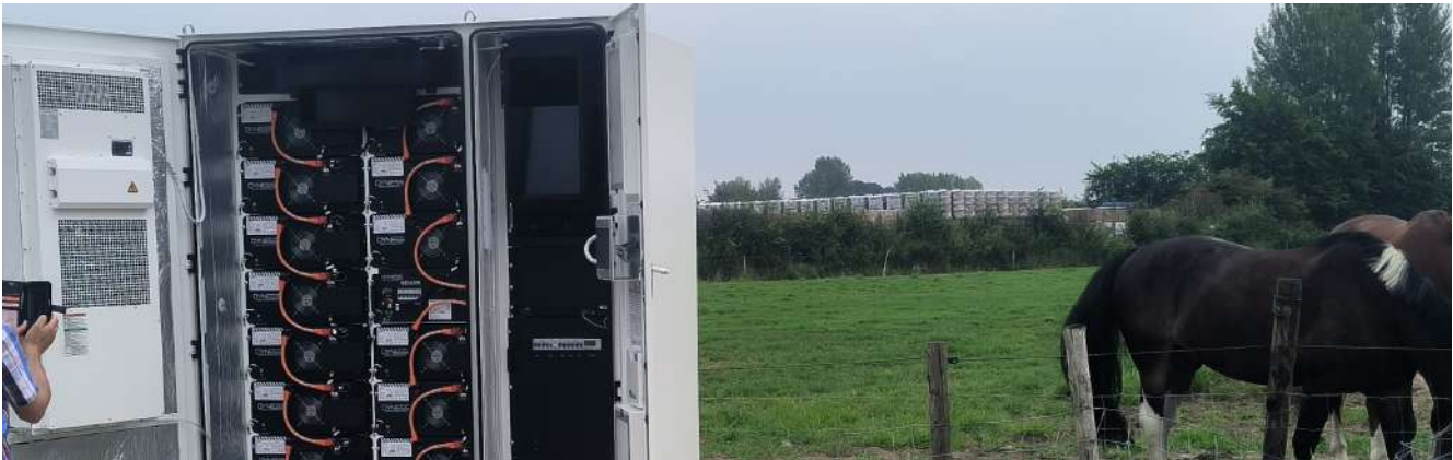
• The Netherlands 100kW/215kWh DH200F PV consumption (self-use)
