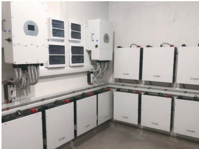
• 48kWh 10 units A48100 Lebanon
