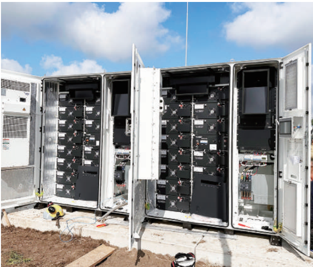
Netherland DH200F 200kW/430kWh Peak-shaving + PV consumption+ Charging pile
