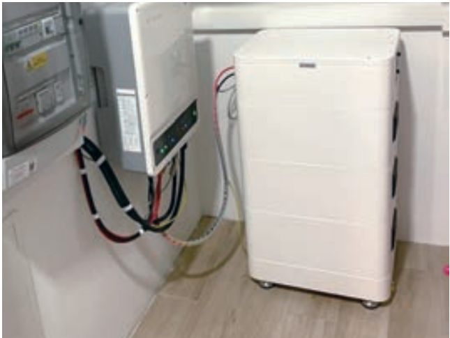
• 10.66kWh Tower T10 Czech Republic
