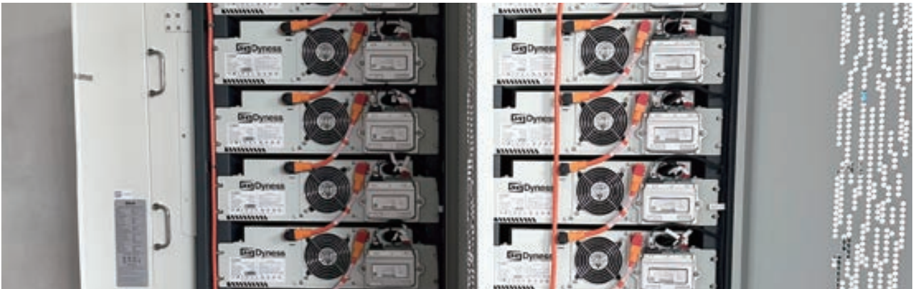
Bulgaria 112.64 kWh PowerRack HV4F Peak-to-valley arbitrage+Self-generation and self-use
