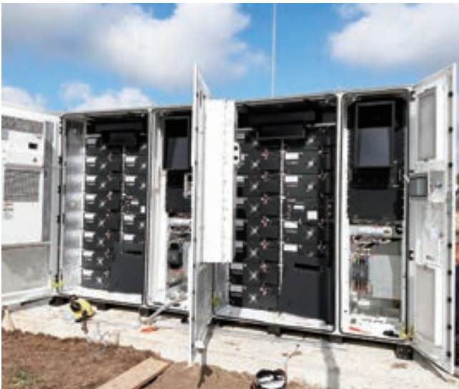
Netherland 300kW/645kWh DH200F Dynamic capacity expansion + PV consumption+ Charging pile
