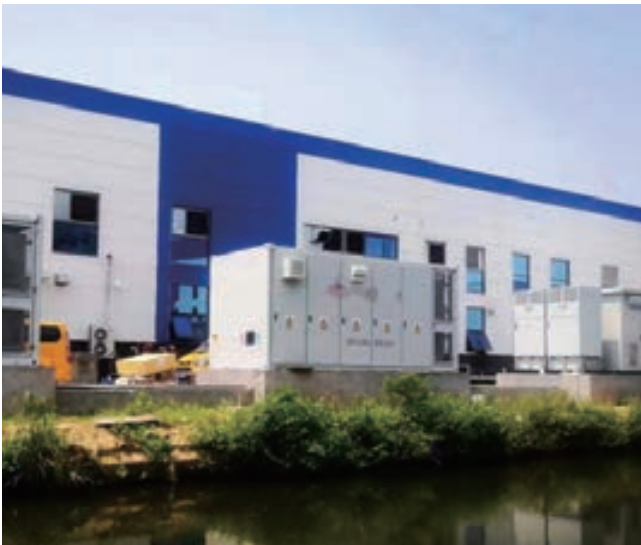
China 5MW/18MWh DH200F Peak-shaving+PV consumption
