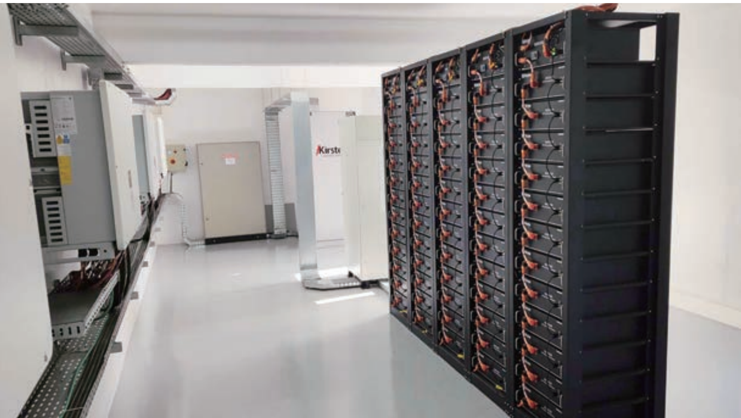
Brazil 100kW/307kWh PowerRack HV4 Dynamic capacity expansion (peak-shaving) + PV consumption
